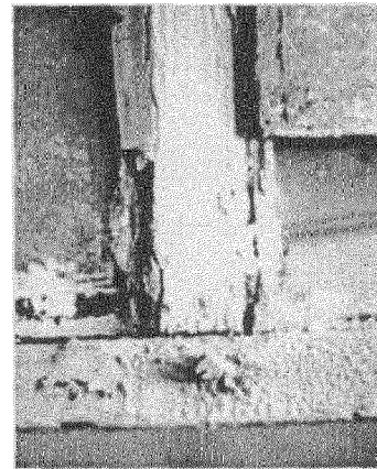
This historic double-hung window has many layers of paint, some cracked and missing putty, slight separation at the joints, broken sash cords, and one cracked pane. Photo: NPS files.
