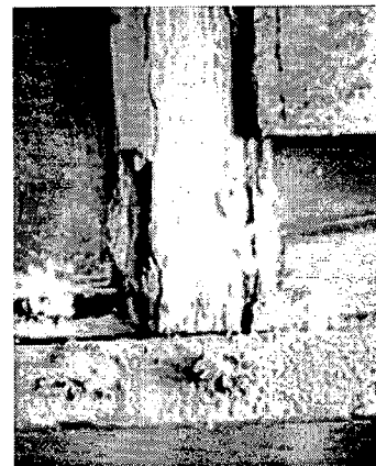
This historic double-hung window has many layers of paint, some cracked and missing putty, slight separation at the joints, broken sash cords, and one cracked pane. Photo: NPS files.
