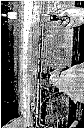
After removing paint from the seam between the interior stop and the jamb, the stop can be pried out and gradually worked loose using a pair of putty knives as shown. Photo: NPS files.
