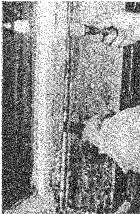
After removing paint from the seam between the interior stop and the jamb, the stop can be pried out and gradually worked loose using a pair of putty knives as shown. Photo: NPS files.
