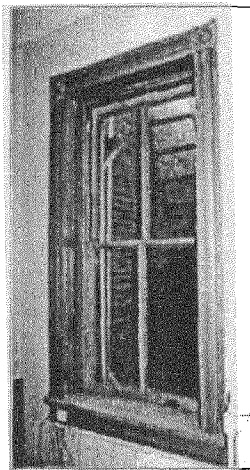
Following the relatively simple repairs, the window is weathertight, like new in appearance, and serviceable for many years to come. Photo: NPS files.
