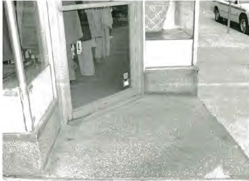
Original gray terrazzo (cracked in corner) and green granite(?) terrazzo kick plates
