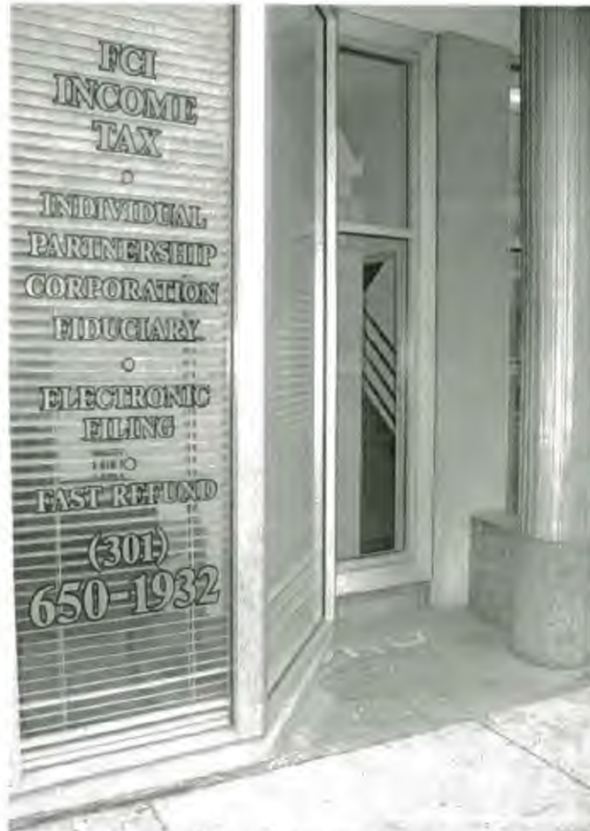
Original aluminum column with partial gray granite terrazzo flooring and newer storefront
