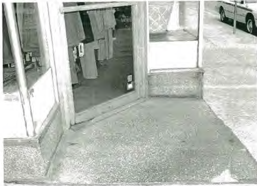
Original gray terrazzo (cracked in corner) and green granite(?) terrazzo kick plates
