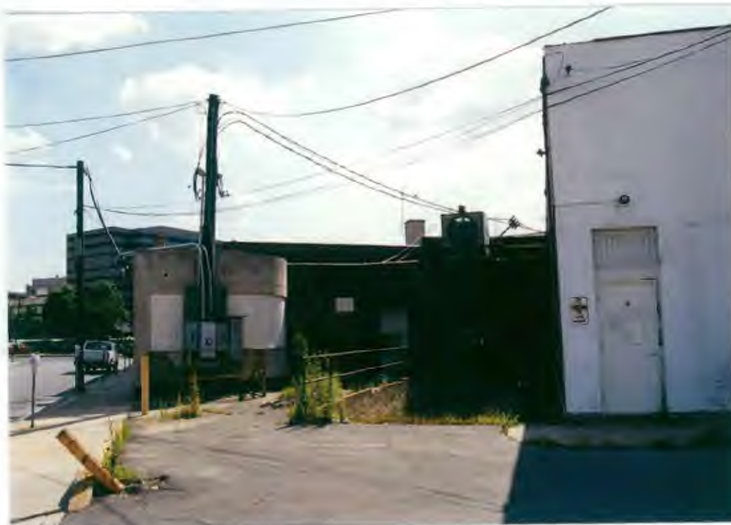
8. DIRECT VIEW OF CURVED END WALL, WHICH THE PROJECT PROPOSES TO BE INCORPORATED WITHIN NEW RETAIL SPACE, BUT VISIBLE THROUGH CLEAR GLAZED STOREFRONT.
