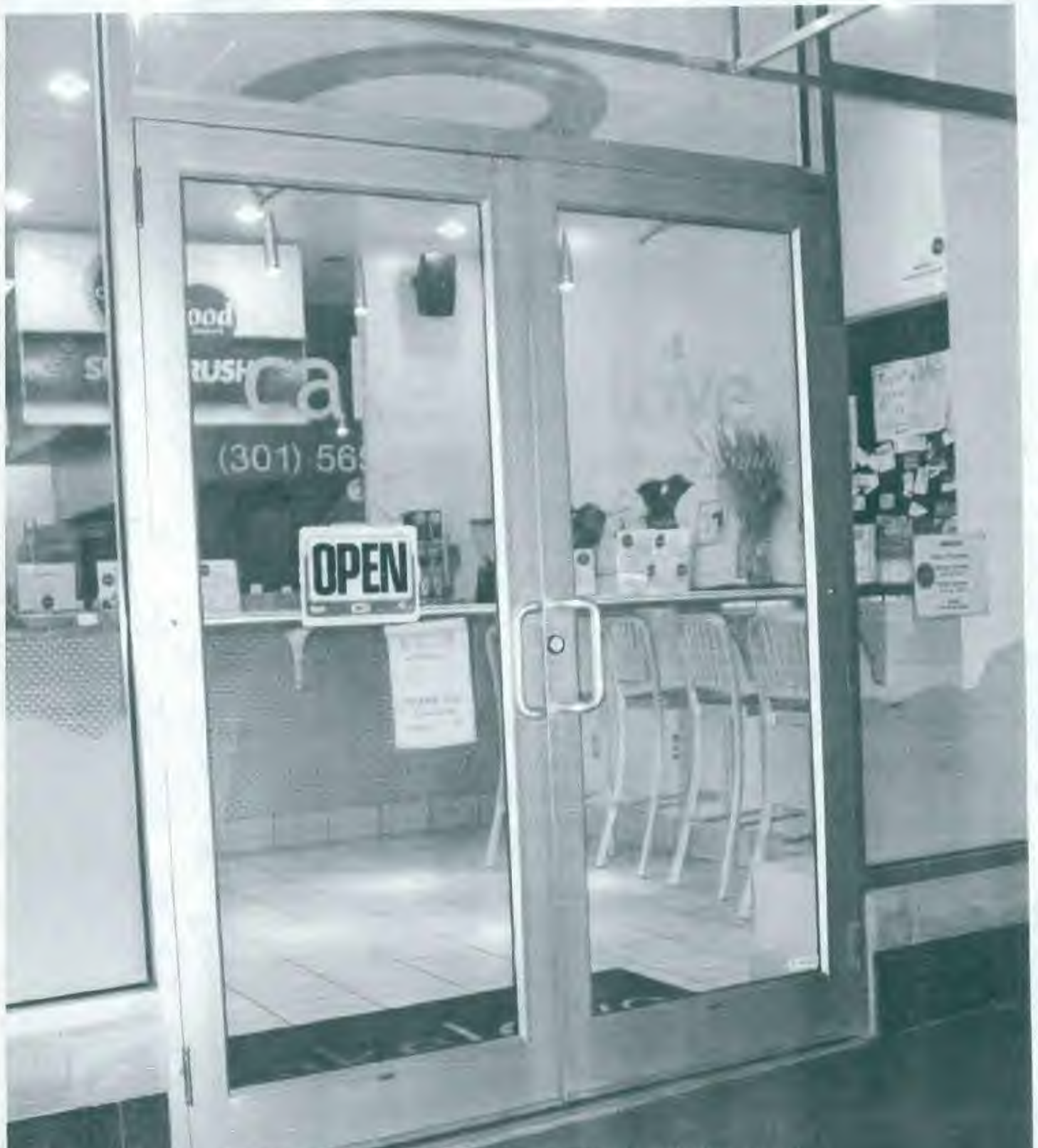
EXISTING "CAKE LOVE" RUSH DOUBLE DOOR ENTRY. PLEASE NOTE THAT THIS ENTRY AND STORE IS NEW WITHIN THE PAST SIX MONTHS!
