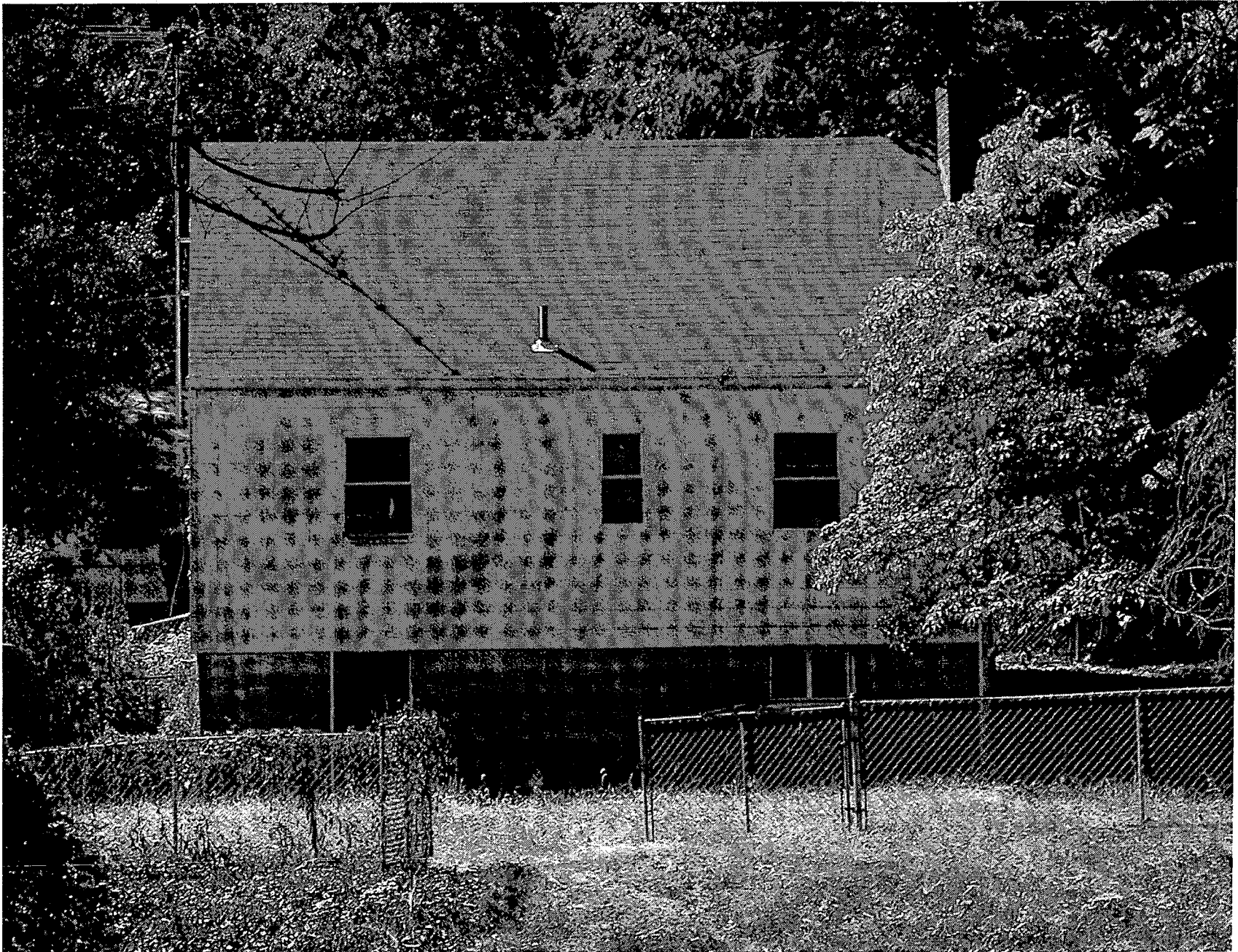
BACK ELEVATION TAKEN FROM 10009 BACK YARD. EXISTING RESIDENCE FROM TOP OF CMU BASEMENT WALL TO BE REMOVED
