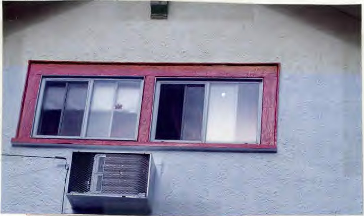
Detail: CLDSE-UP of ALUMINUM WINDOWS TO BE REPLACED
