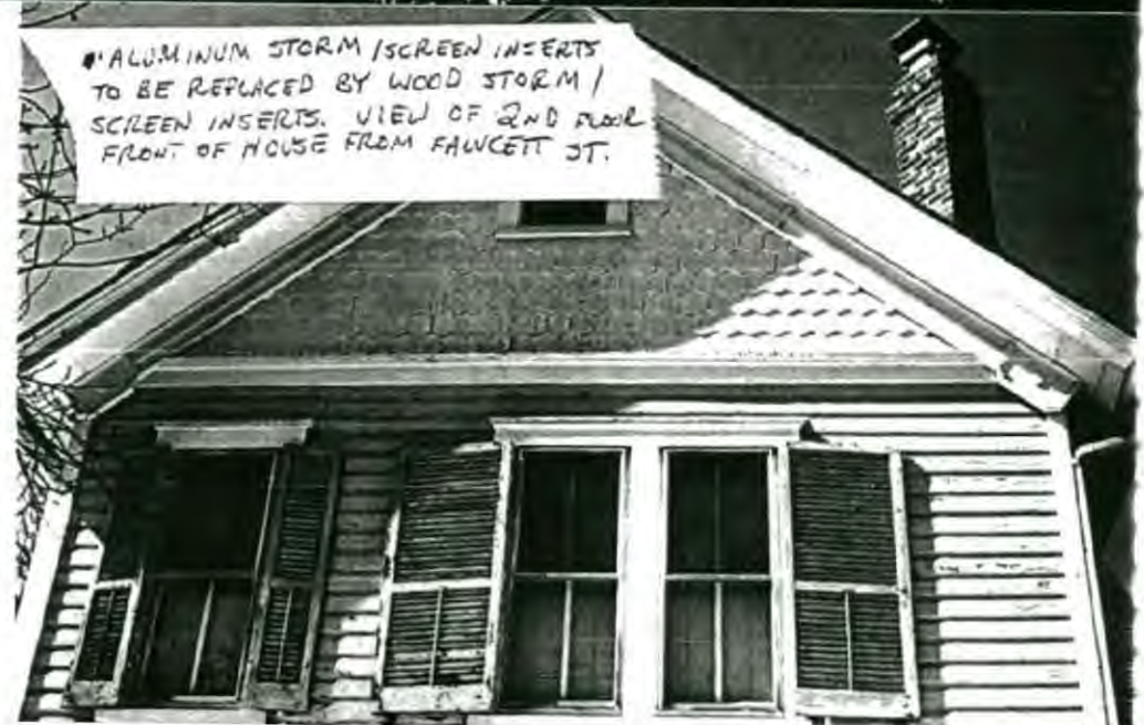
ALUMINUM STORM / SCREEN INSERTS TO BE REPLACED WITH WOOD STORM / SCREEN INSERTS. VIEW OF 2ND FLOOR SOUTH SIDE OF HOUSE FROM NEIGHBOR'S YARD.
