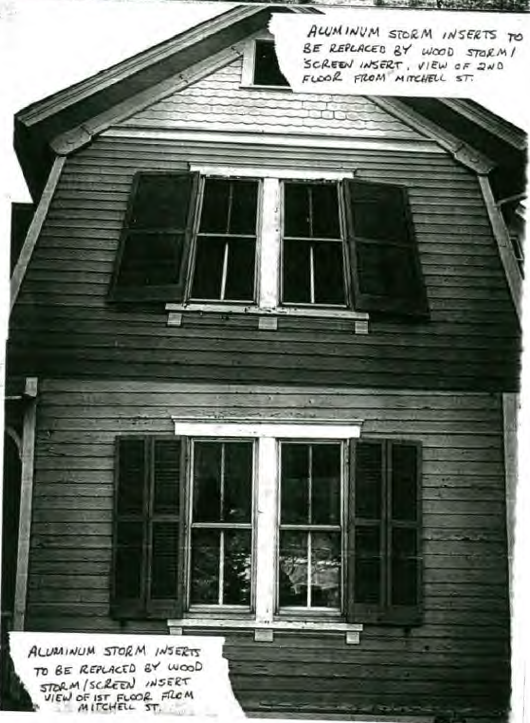
REPLACE ALUMINUM STORM INSERTS WITH WOOD STORM/ SCREEN INSERTS. VIEW OF 1ST FLOOR FRONT OF HOUSE FROM FAWCETT ST.
