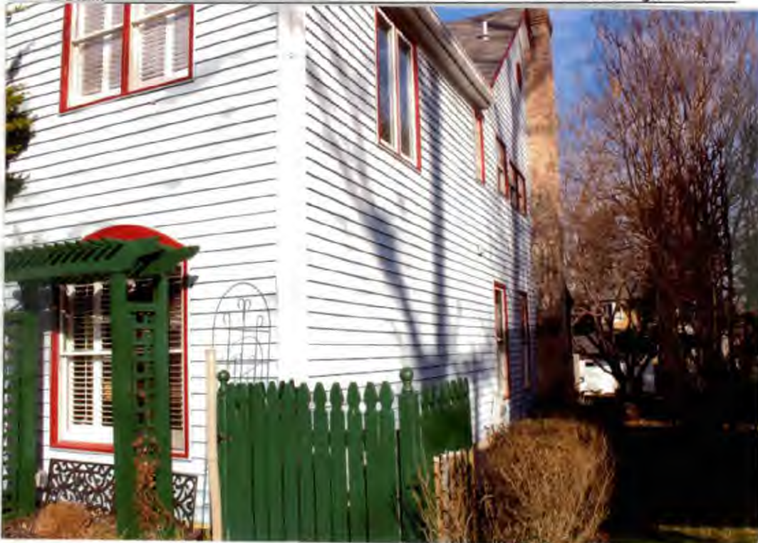
Detail: Looking down south-facing side of house. there is only a 3-FT setback from neighbor's property so the picture is angled
