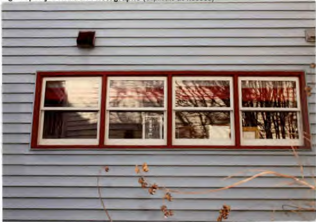
Detail: North facing windows - all w/ rotted wood.
