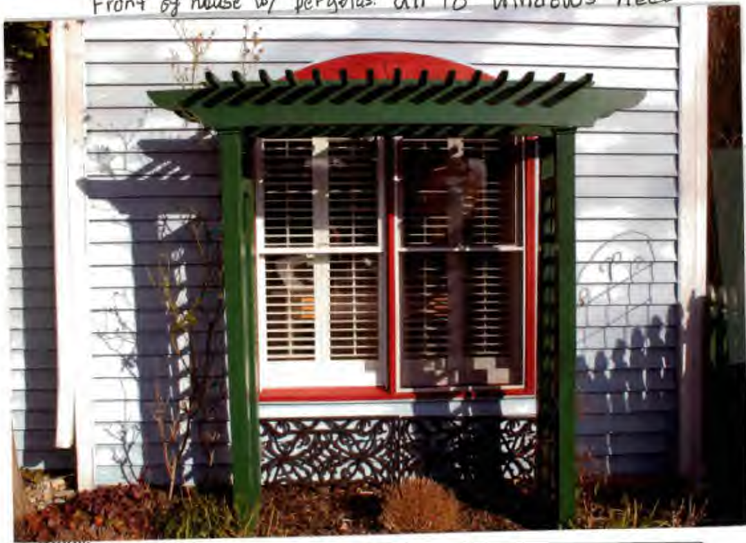
to be replaced - 4 up, 6 down - from rain and moisture damage
