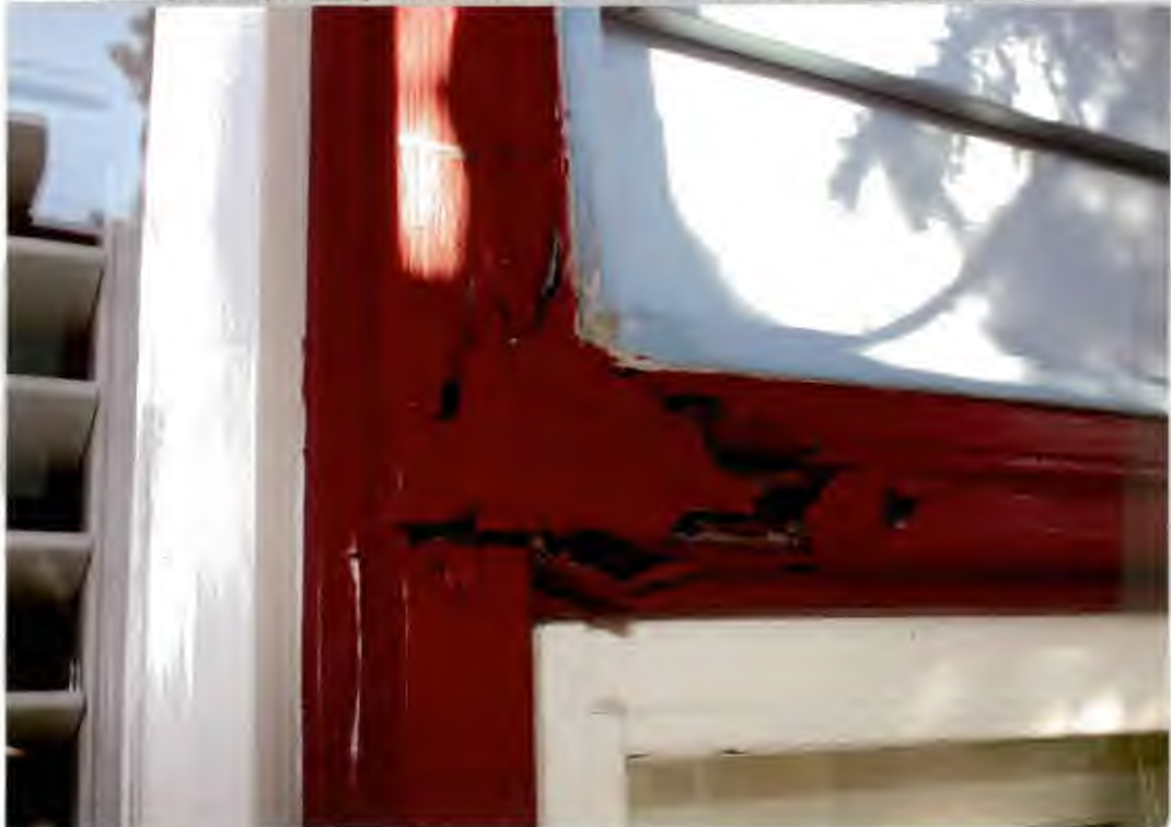
Detail: Example of window damage in front
