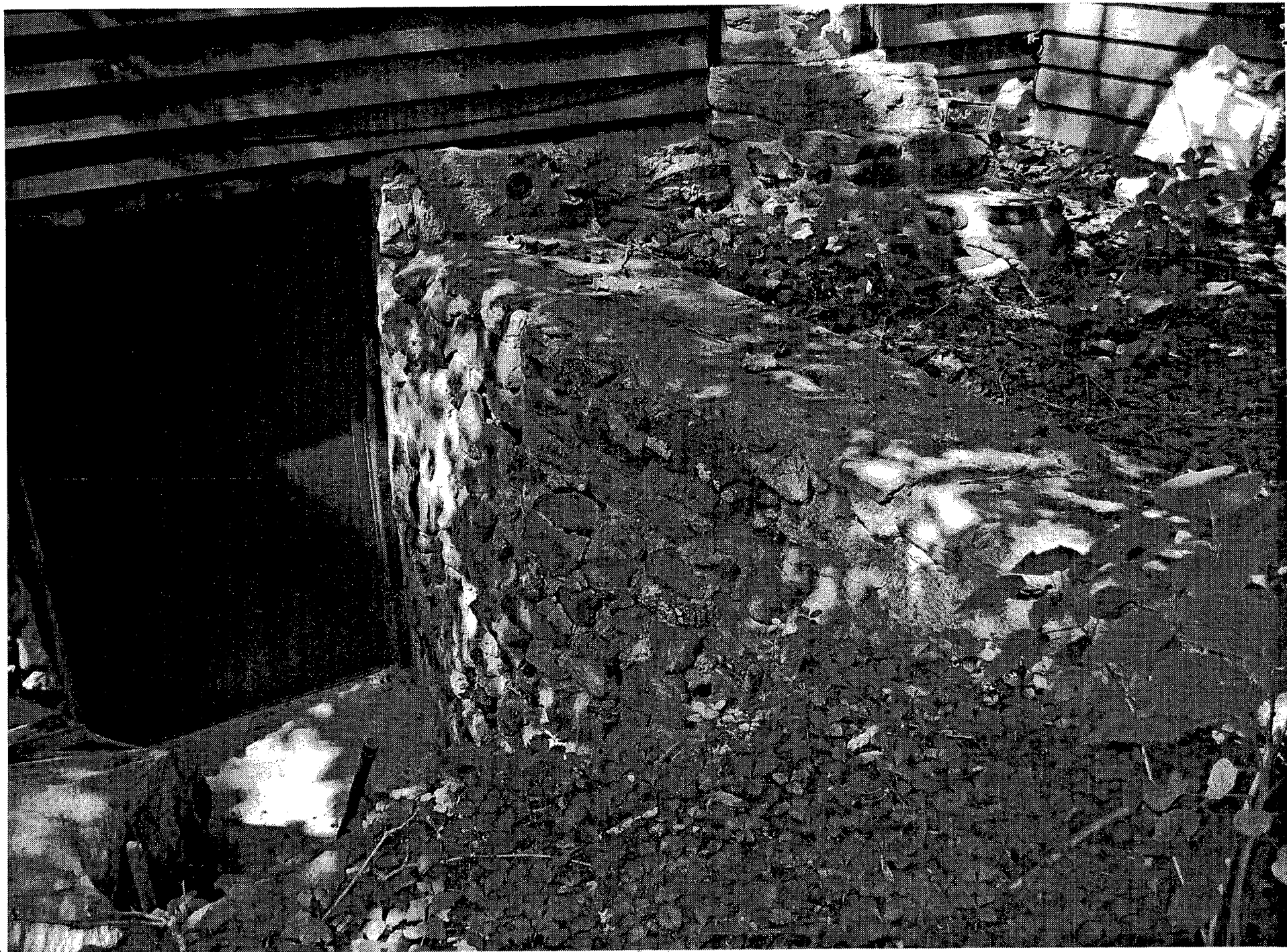
28 WALL B + CELLAR DOOR, ALSO OLD SHED LAUNDRY ROOM FOUNDATION -
