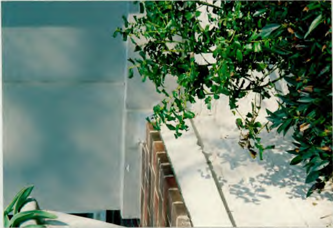
Detail: MISSING BRICK @ WALL CAP
