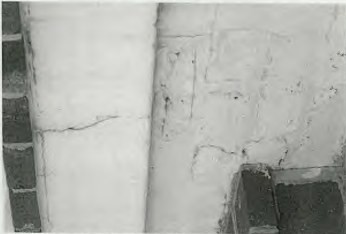
Detail: CRACKED CONC CAP BELOW BRICK TOP @ END WALLS.
