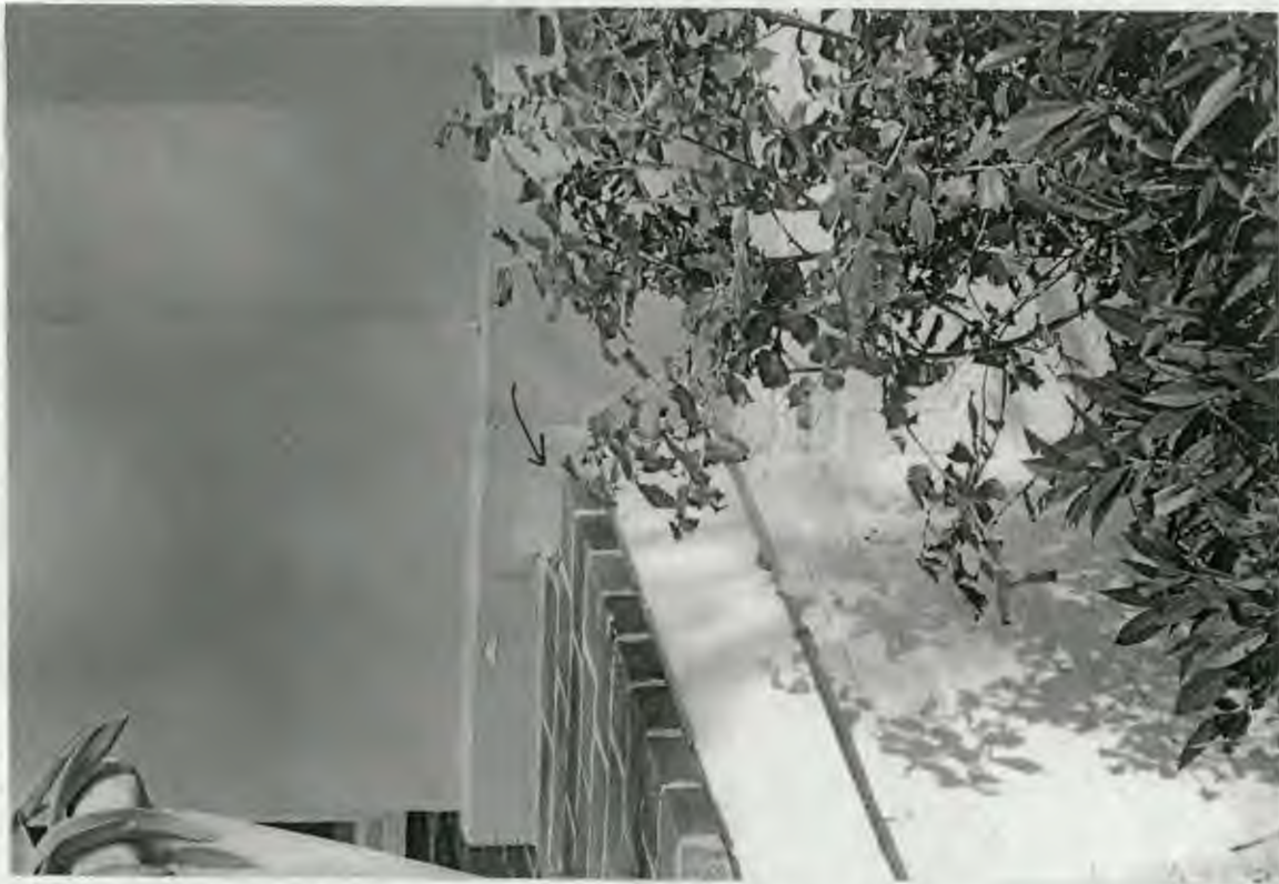
Detail: MISSING BRICK @ WALL CAP
