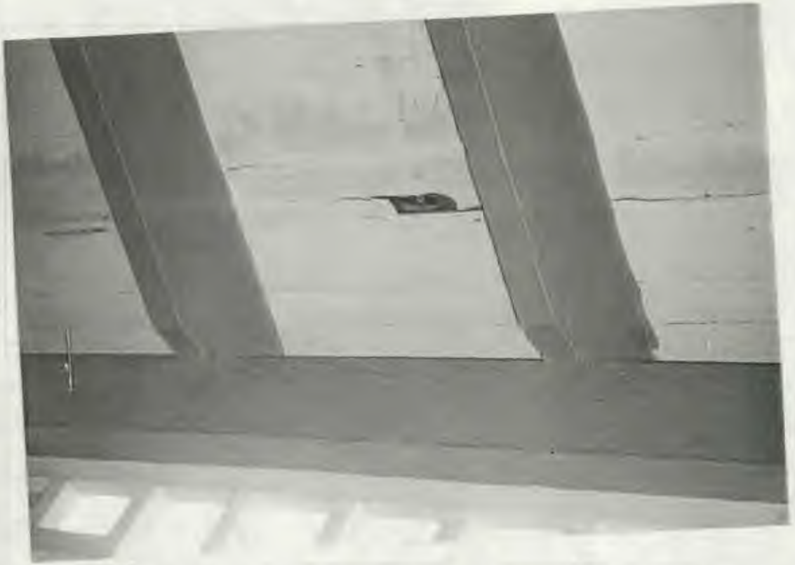
UNDERSIDE OF PORCH ROOFING SHOWING DETEIORATION CAUSED BY LEAKING ROOF FLASHING
