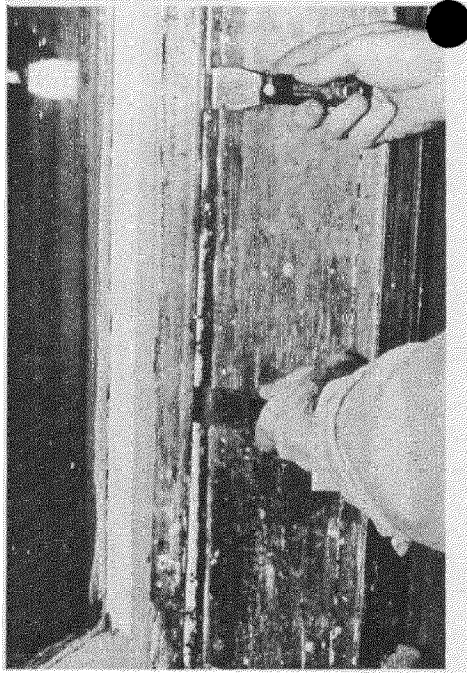
Figure 4b. After removing paint from the seam between the interior stop and the jamb, the stop can be pried out and gradually worked loose using a pair of putty knives as shown. To avoid visible scarring of the wood, the sash can be raised and the stop pried loose initially from the outer side: Photo: John H. Myers
