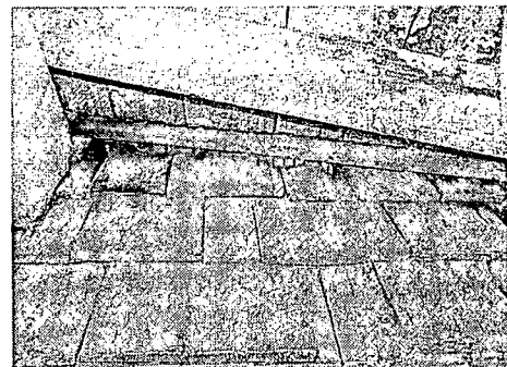
Shakes within leanto showing non-weathered condition
