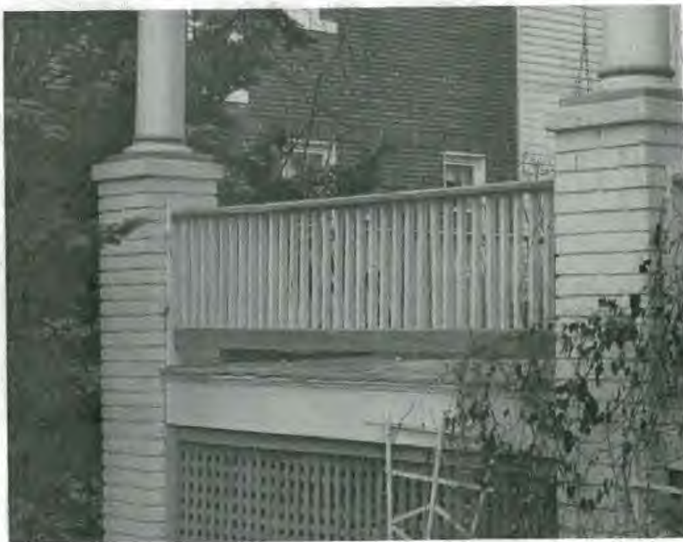
Picture #7 – Detail of front porch – new rear porch will match railing, lattice, and skirt
