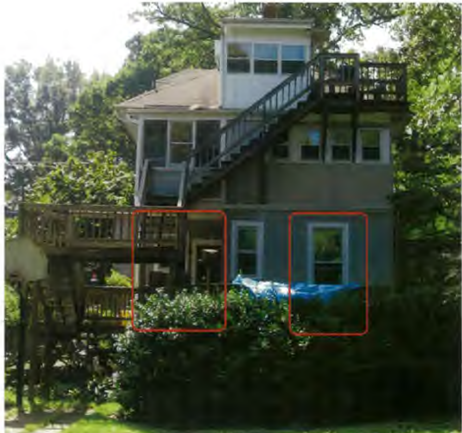
view of northwest face from backyard (area of infill addition at left, area of bay addition at right)
