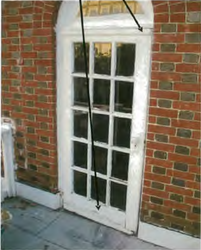
Attempted repairs, original wood style
