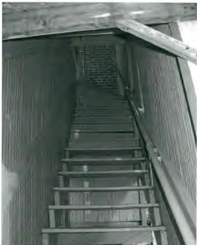
7102 Steps, very steep Some pieces missing and loose/deteriorating
