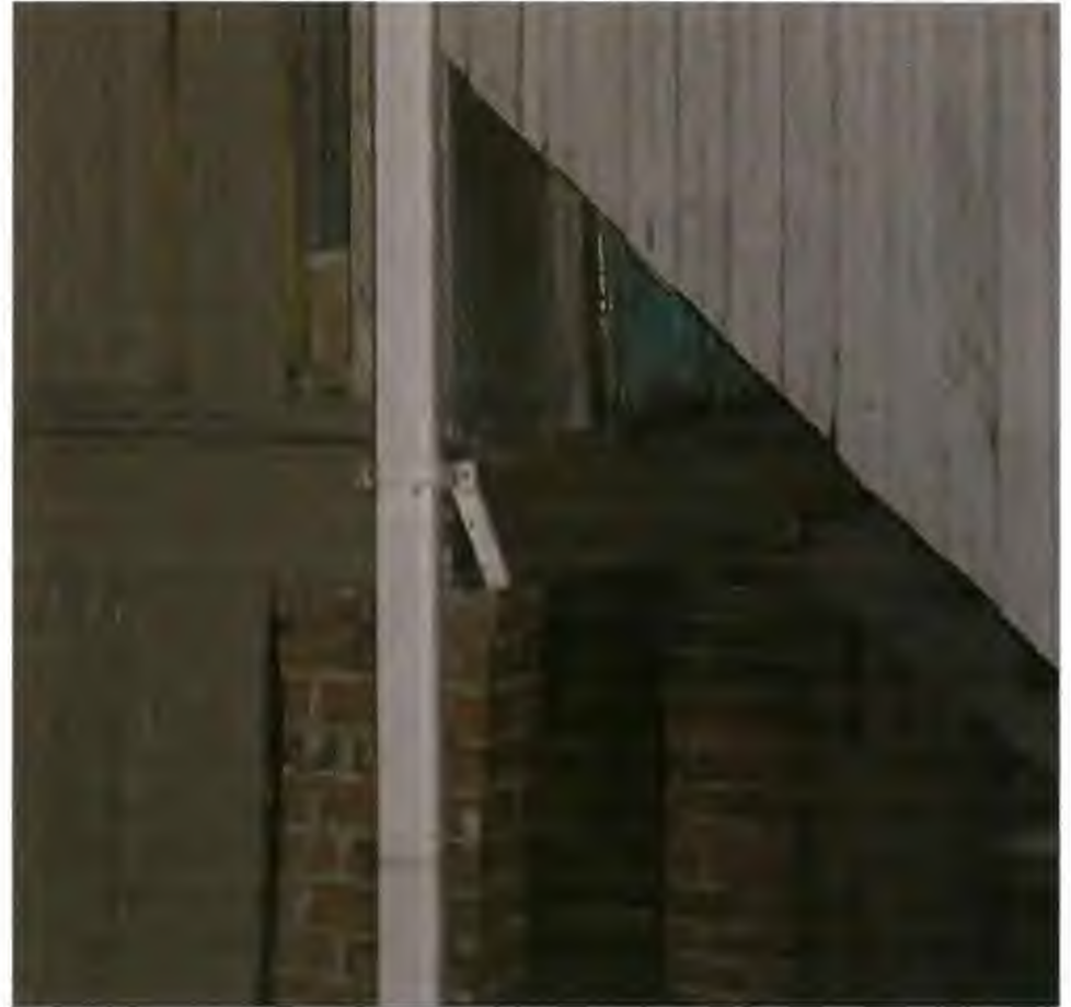
Twisted support on 7104 side Notice leaning pier, too
