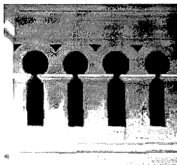
The paint on this exterior decorative feature is sound. Photo: NPS files.
