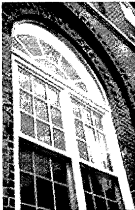
When the paint on the wood windows became too thick, it was removed and the window repainted. Photo: NPS files.
