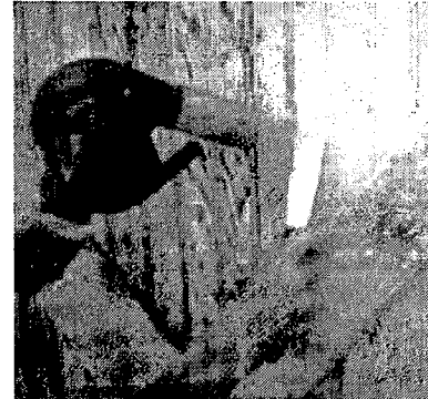
The nozzle on the electric heat gun permits hot air to be aimed into cavities on solid decorative surfaces, such as this carriage house door. After the paint has been sufficiently softened, it can be carefully removed with a scraper. Photo: NPS files.
